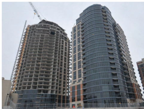
Sierra and Palomar make up the final phase of Village Gate West
